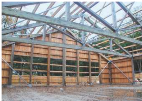
The new Machinery Store is constructed from massive timbers and now ready for the roof
